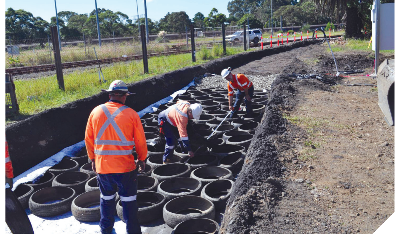
According to Oxford Economics Australia, there has been a substantial rise in the construction and maintenance of railways in Australia, reaching an all-time high of $12.9 billion in 2021-22. Source: Buddhima Indraratna
