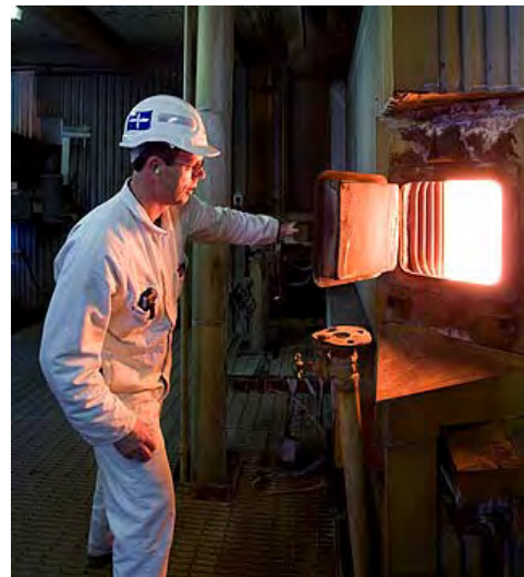
Figure 3 Opening an inspection door in a furnace (called a boiler) at Loy Yang Power Station in Victoria. The fuel being burnt is coal. The furnaces in which the coal is burnt are almost as high as a 12-storey building!
